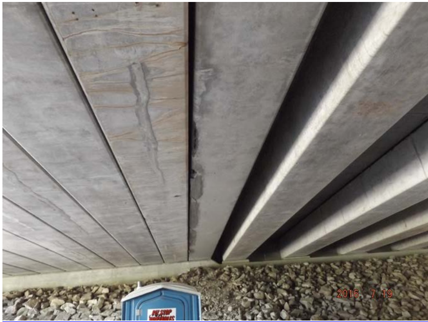
SPAN 4 - BEAM L - REBAR SPALLS
