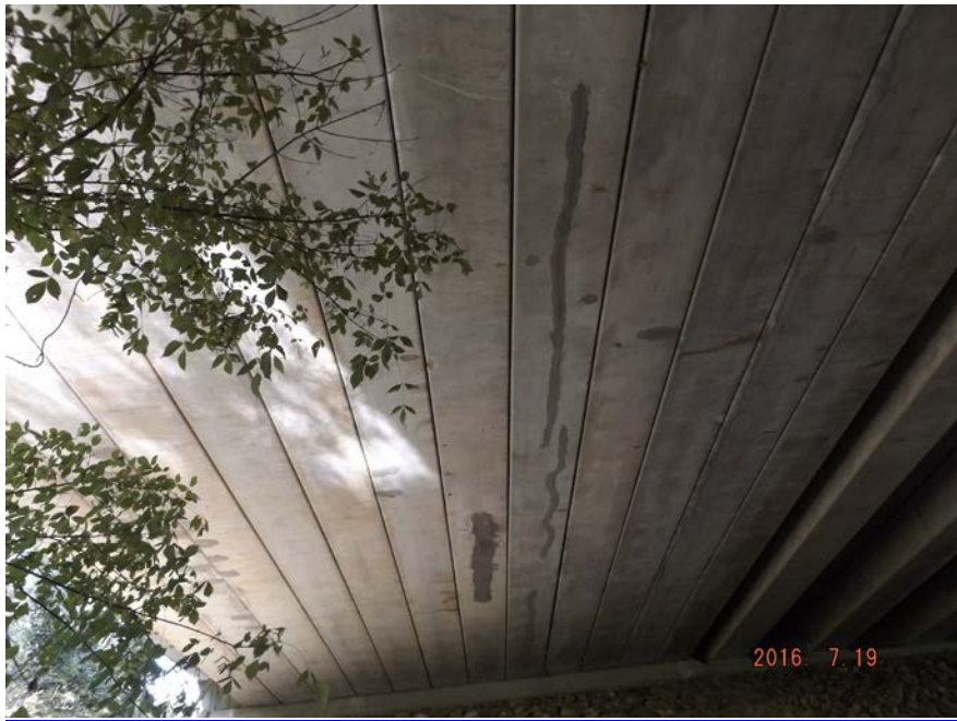
SPAN 1 - LEFT - PATCHED CRACKS/DELAMS
