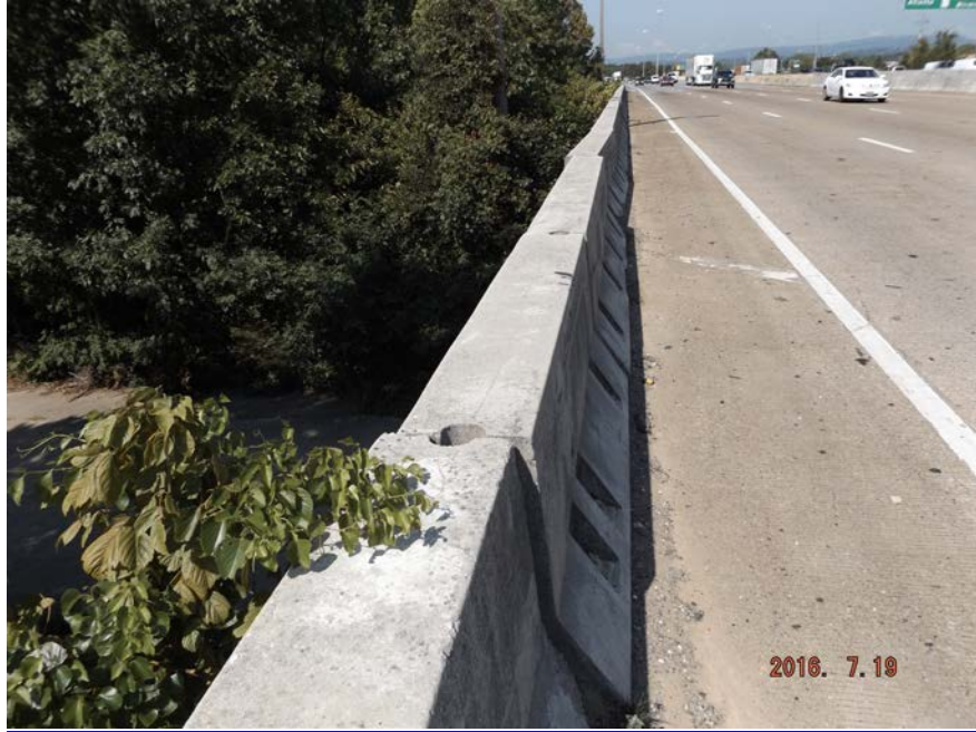
SPAN 4 - RIGHT - BRIDGE RAIL - COLLISION DAMAGE
