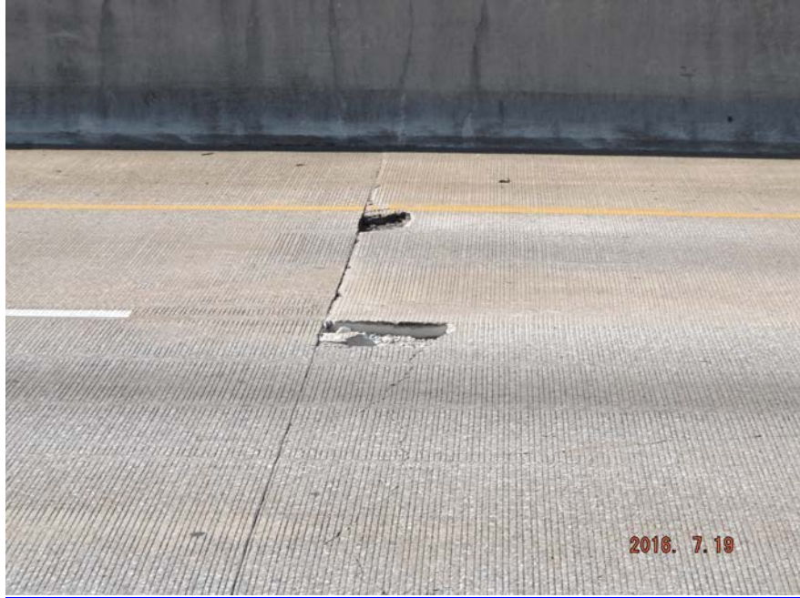
APPROACH 1 - SB - POTHOLE
