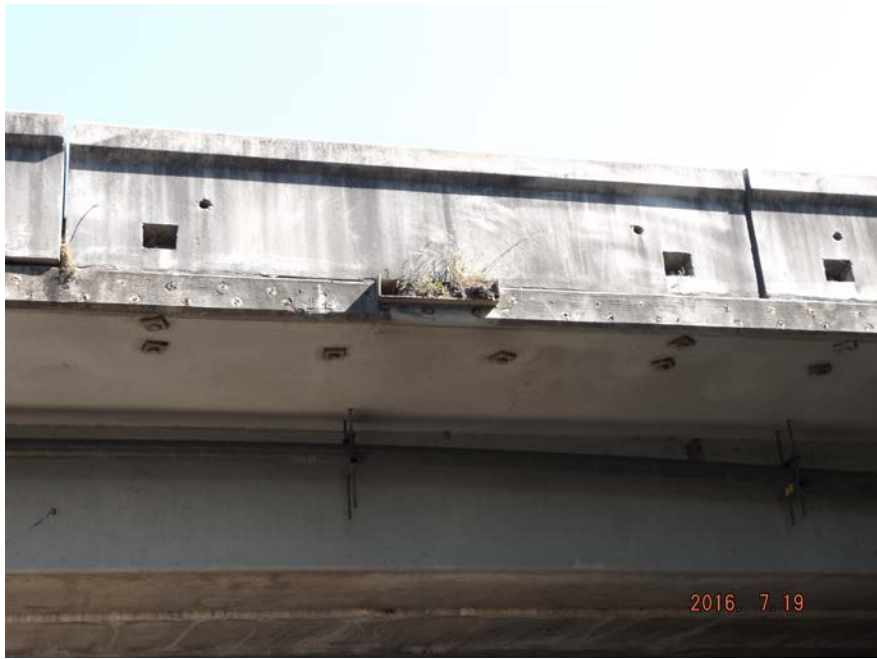
SPAN 4 - RIGHT - DRAIN CLOGGED
