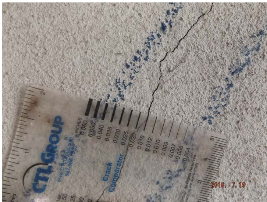
SPAN 4 - BEAM A - ABUTMENT 2 - SHEAR CRACK
