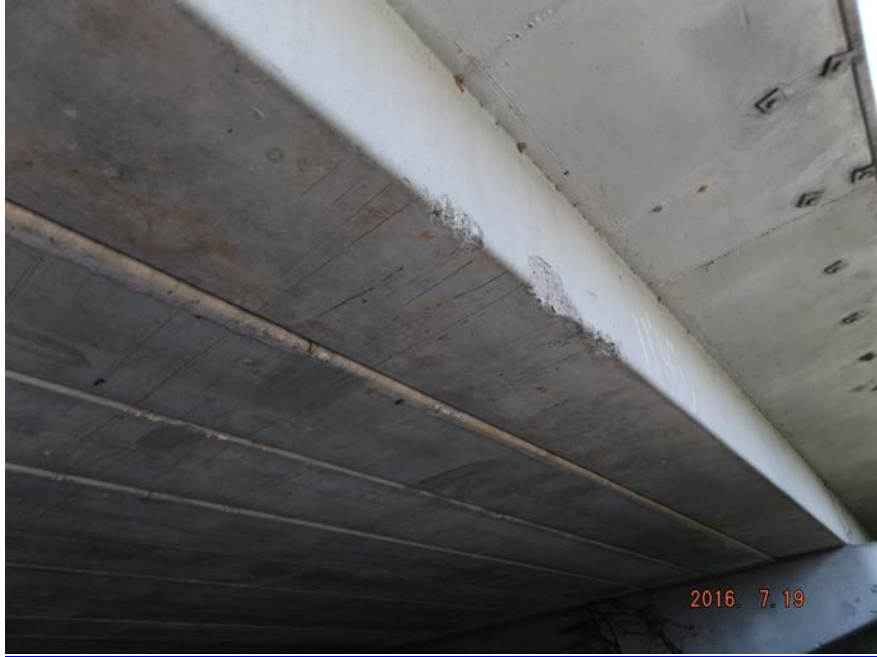
SPAN 4 - BEAM A - MID SPAN - SPALLS
