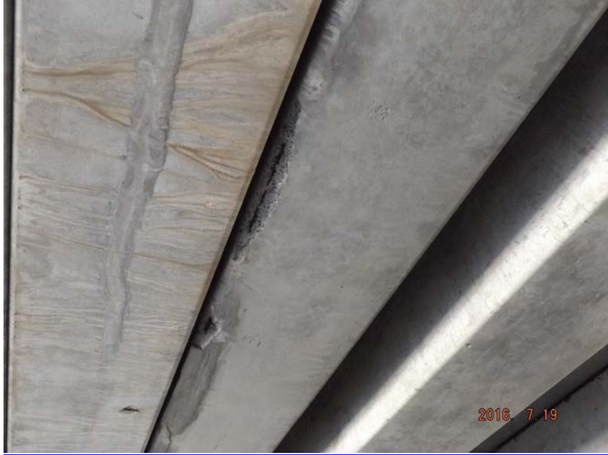
SPAN 4 - BEAM L - REBAR SPALLS
