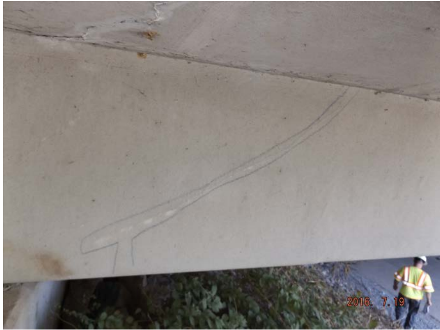
SPAN 4 - BEAM A - ABUTMENT 2 - SHEAR CRACK
