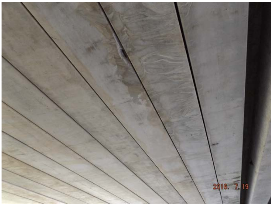
SPAN 3 - BEAM U - REBAR SPALL
